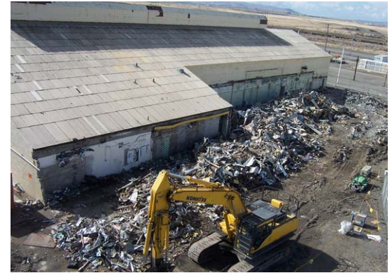
The 314 Building in the 300 Area is one of the more than 500 excess Hanford facilities D4 Closure Project workers will demolish during the River Corridor Closure Project.
