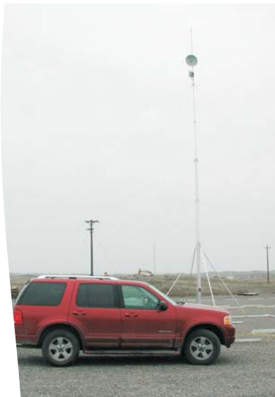
Wireless tower in place at the 100 N Area. The towers provide network services to remote sites.
