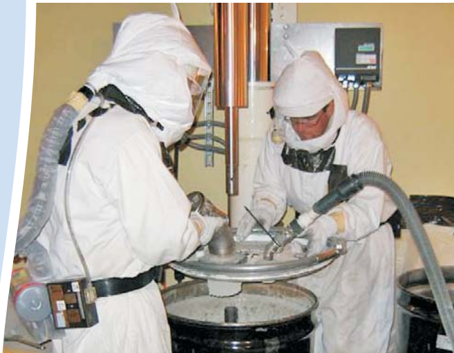
Subcontract workers remove a specially designed lid from a grouted resin waste drum. Workers used an industrial mixer to mix concrete, fly ash and slag with resin and water according to their approved treatment plan for disposal at ERDF. The lid allowed workers to seal the drum and contain the waste in a safe and controlled manner.
