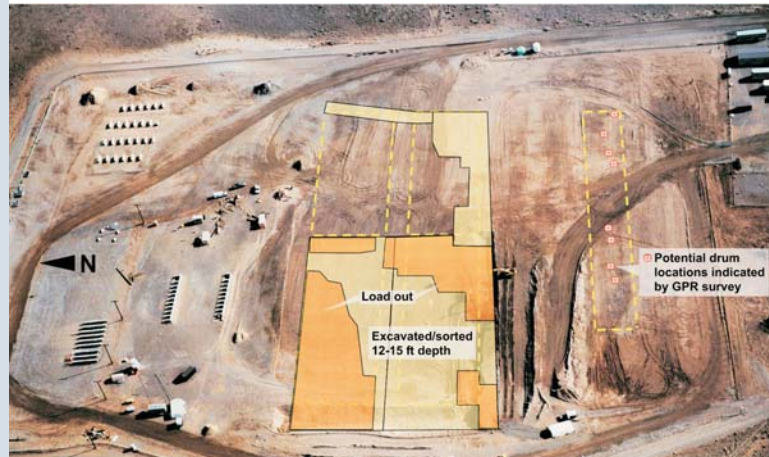
The 618-7 Burial Ground brings unknown challenges in the form of lead debris.
