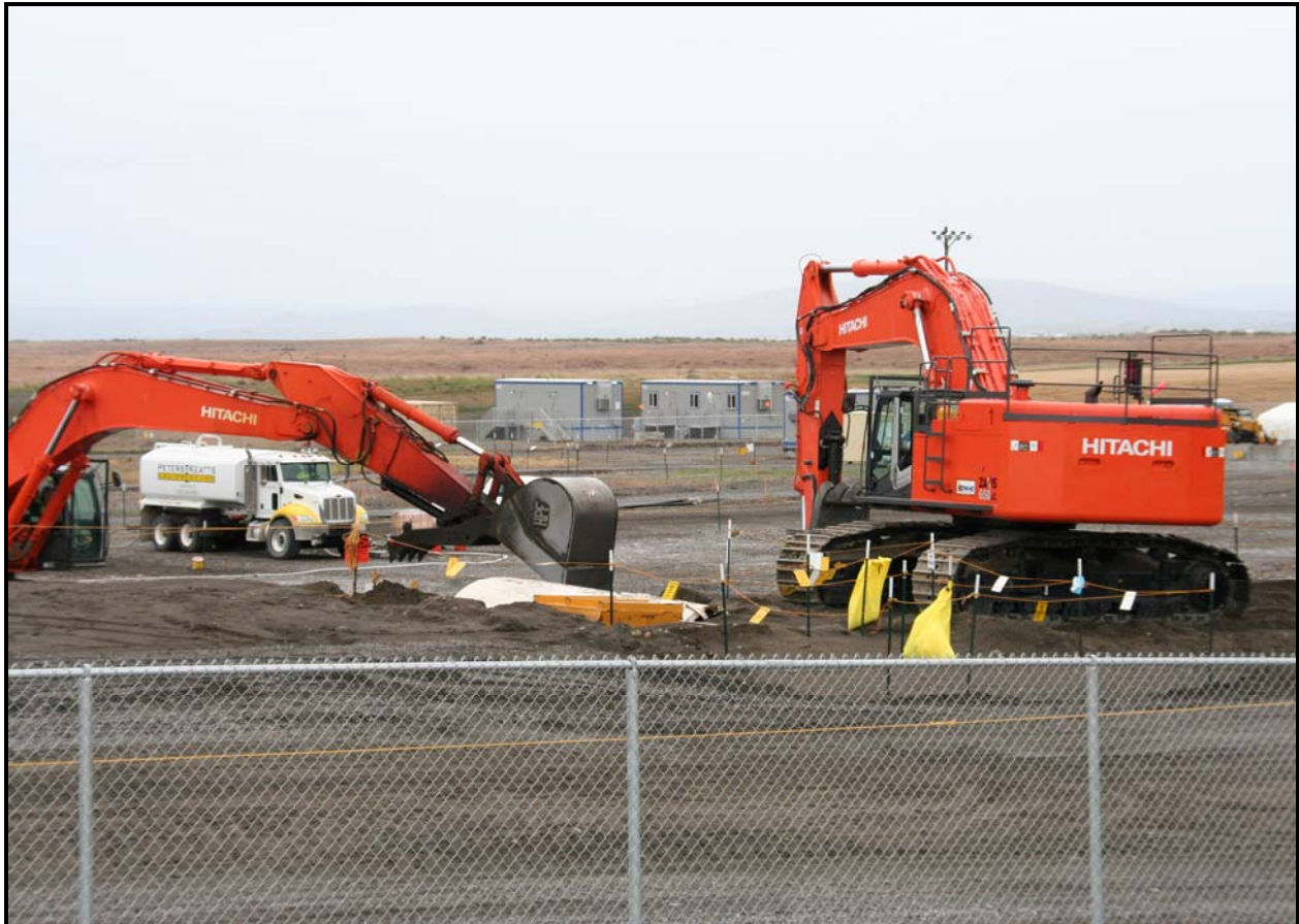
Washington Closure Hanford workers uncover a large steel tank in the north central section of the 618-10 Burial Ground. (Photo 6)
