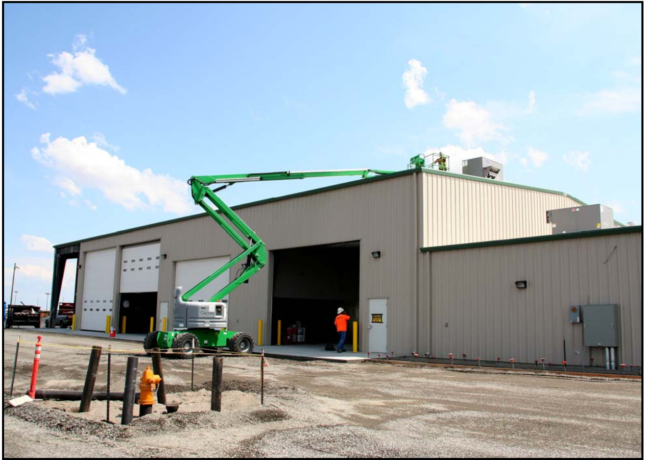
Washington Closure Hanford subcontractor ELRFowler works on an air conditioning unit at the equipment maintenance facility/operations center. (Photo 4)
