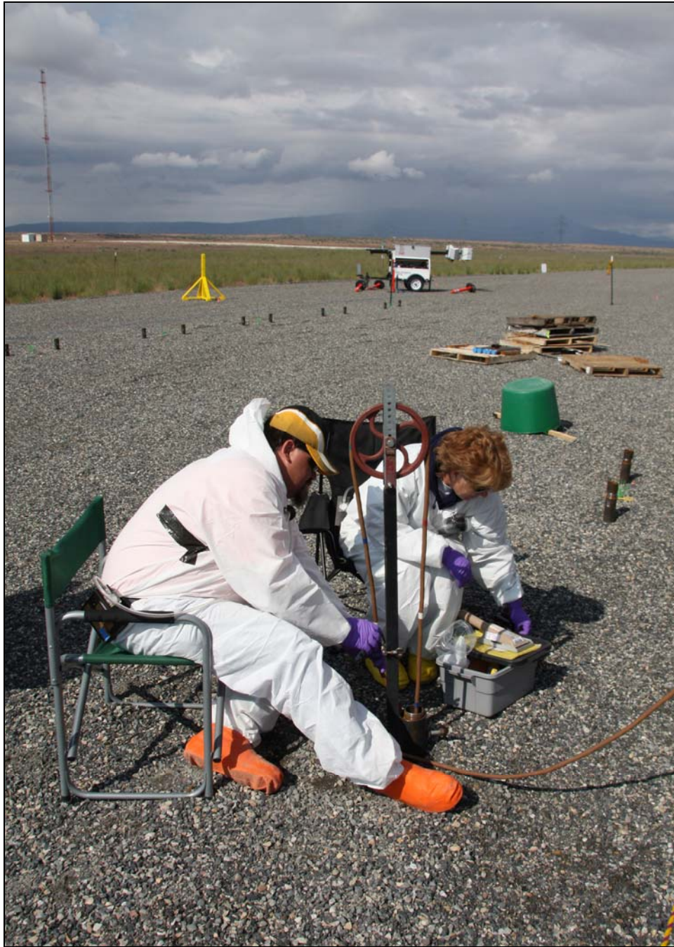
Employees with Washington Closure Hanford and subcontractor North Wind Inc. retrieve a multi-detector probe from a cone penetrometer during nonintrusive characterization of the 618-11 Burial Ground. (Photo 8)
