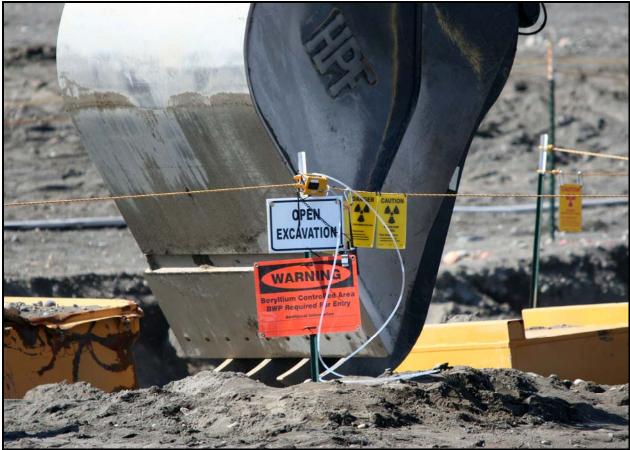
So far, the project team has encountered several drums, including one concreted drum and another containing oil and miscellaneous debris. (Photo 7)
