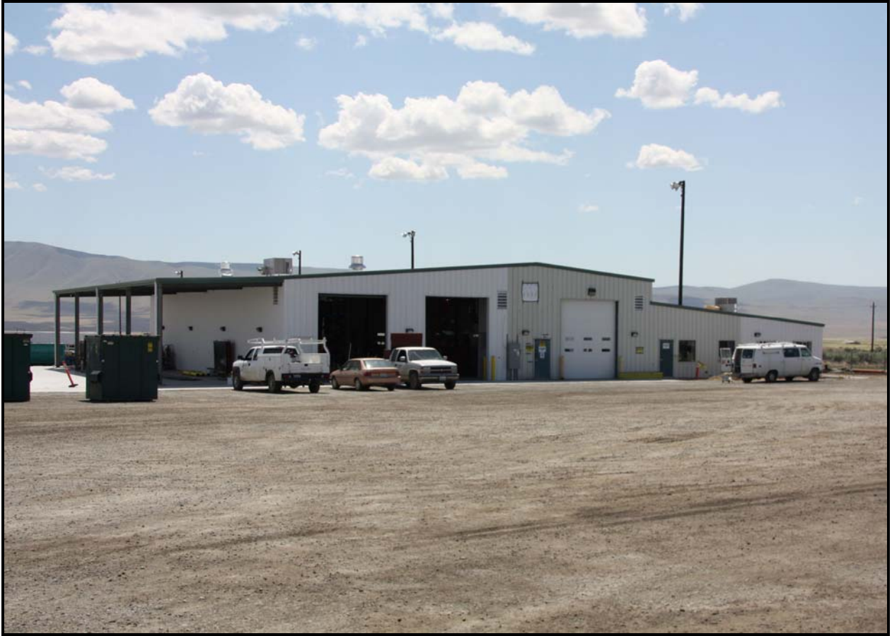
Washington Closure Hanford subcontractor DelHur Industries continues to expand ERDF's transportation maintenance facility. Work on the facility is expected to be completed next month. (Photo 3)
