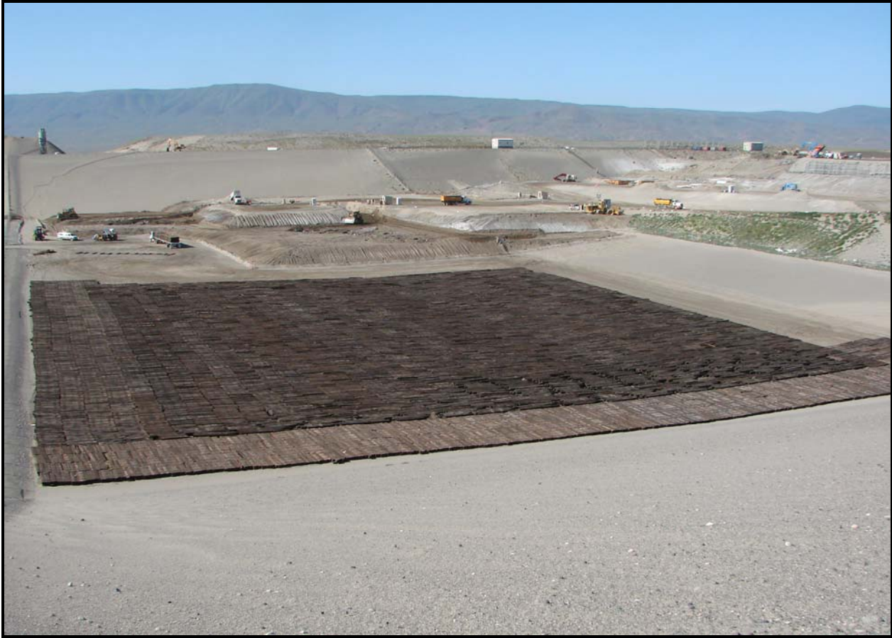
Railroad ties from the Hanford Site continue to be disposed in super cell 9. ERDF is expected to receive nearly 60,000 railroad ties. (Photo 2)
