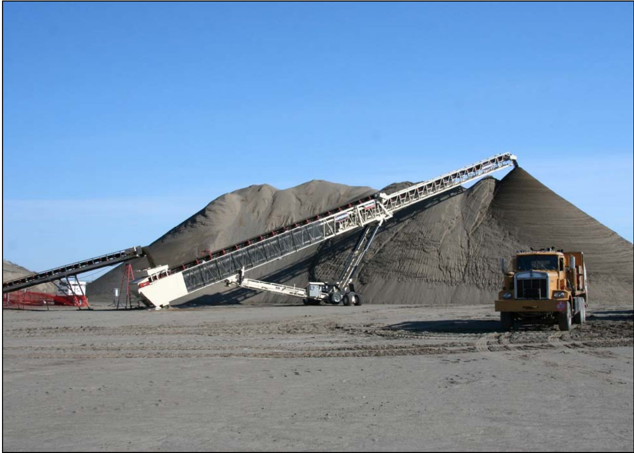
Sand for ERDF's new batch plant continues to be stockpiled. The batch plant will be used to manufacture grout for disposal operations. (Photo 4)
