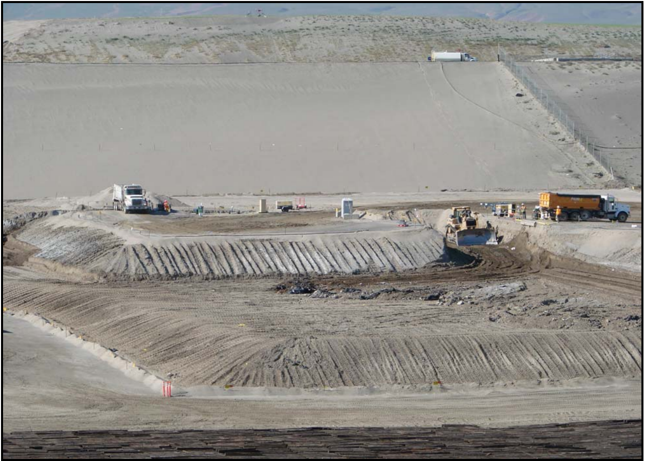
Waste disposal continues in super cell 9 at the Environmental Restoration Disposal Facility. (Photo 1)
