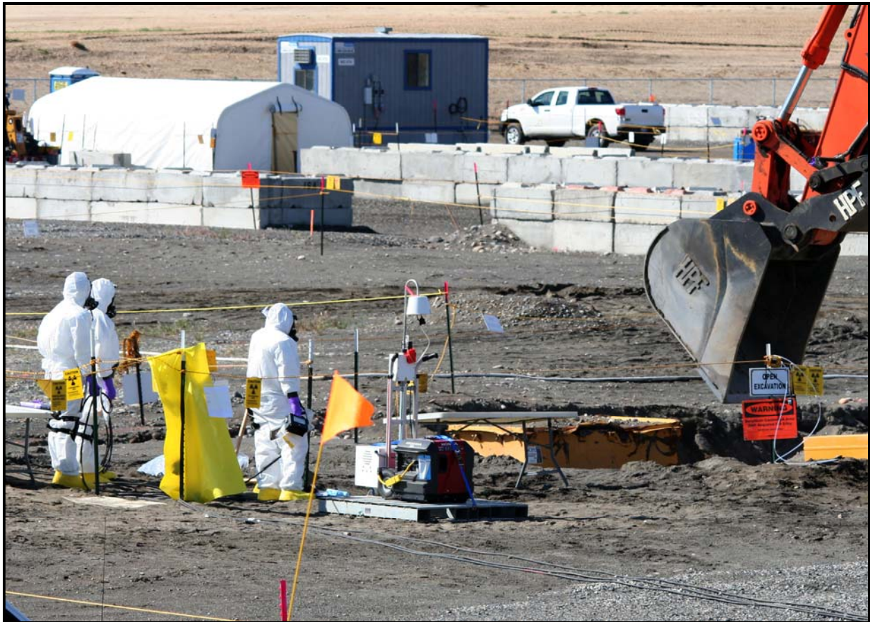
Washington Closure Hanford continues excavation of the waste trenches at the 618-10 Burial Ground. (Photo 6)
