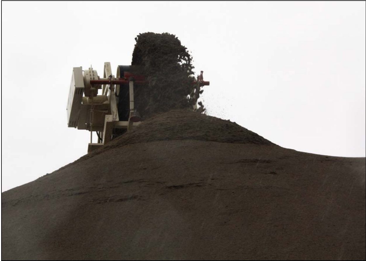
The screen plant continues to stockpile sand for ERDF's new batch plant. Washington Closure Hanford began operational testing of the batch plant last week. (Photo 5)
