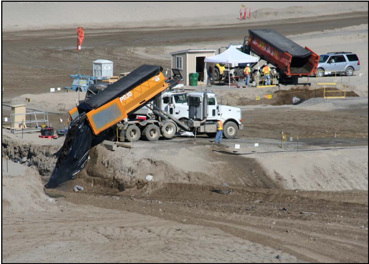
Waste is disposed off two dumps ramps set up in super cell 9 at the Environmental Restoration Disposal Facility. (Photo 2)
