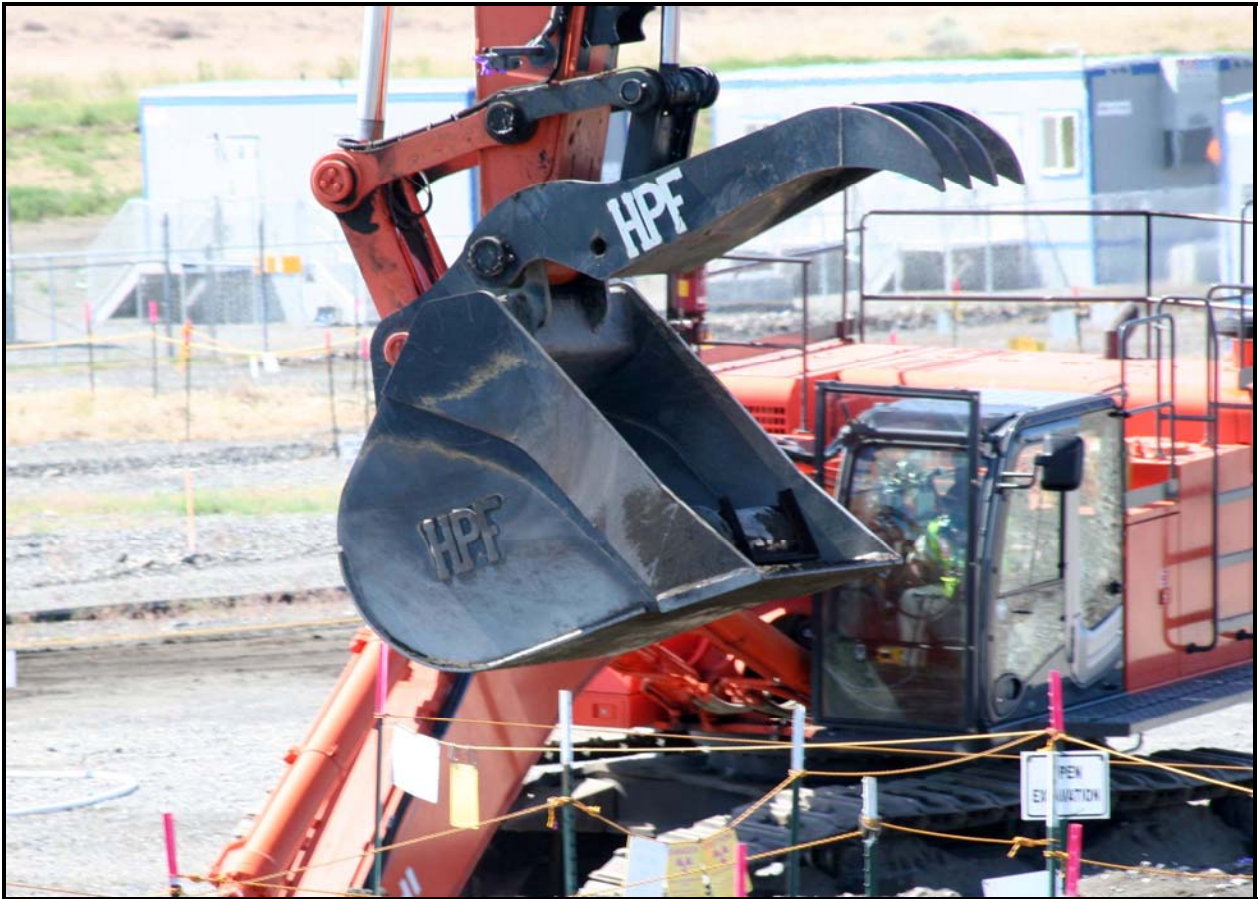
Workers at the 618-10 Burial Ground have been encountering liquid-filled bottles, concrete drums, containers of ion exchange resins, and miscellaneous debris. (Photo 8)
