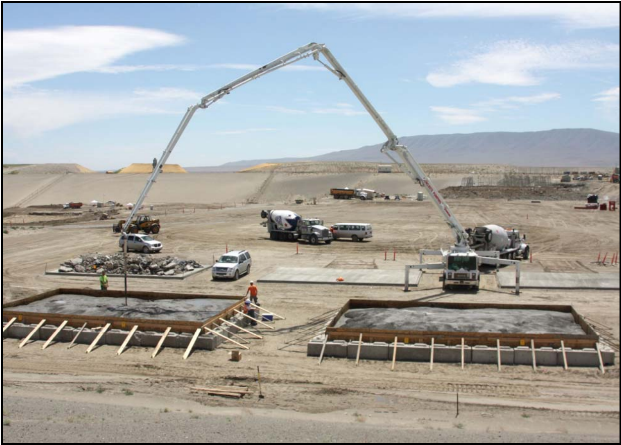
The Waste Operations team at ERDF constructed macro pads to dispose of chromium-contaminated debris. (Photo 5)
