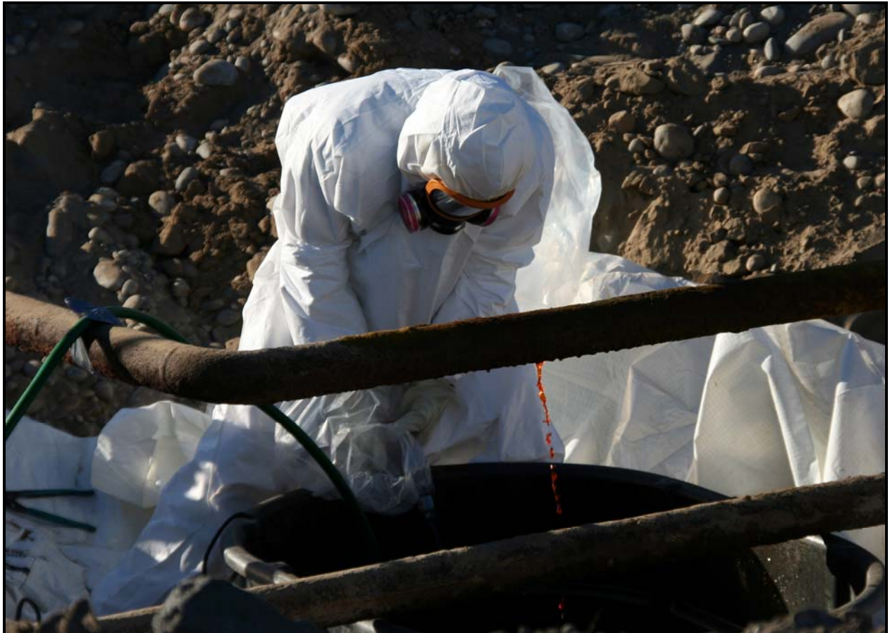
In February, a Washington Closure Hanford subcontractor safely drained sodium dichromate from a pipe at 100-F-26:7. (Photo 8)
