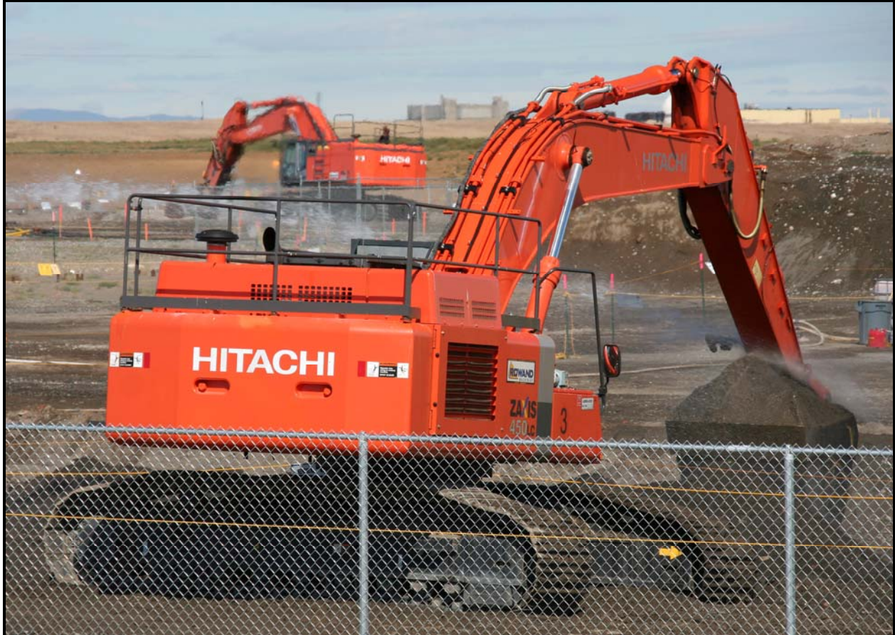
Excavation of the waste trenches continues at the 618-10 Burial Ground. The project team is working in the south trench. (Photo 5)
