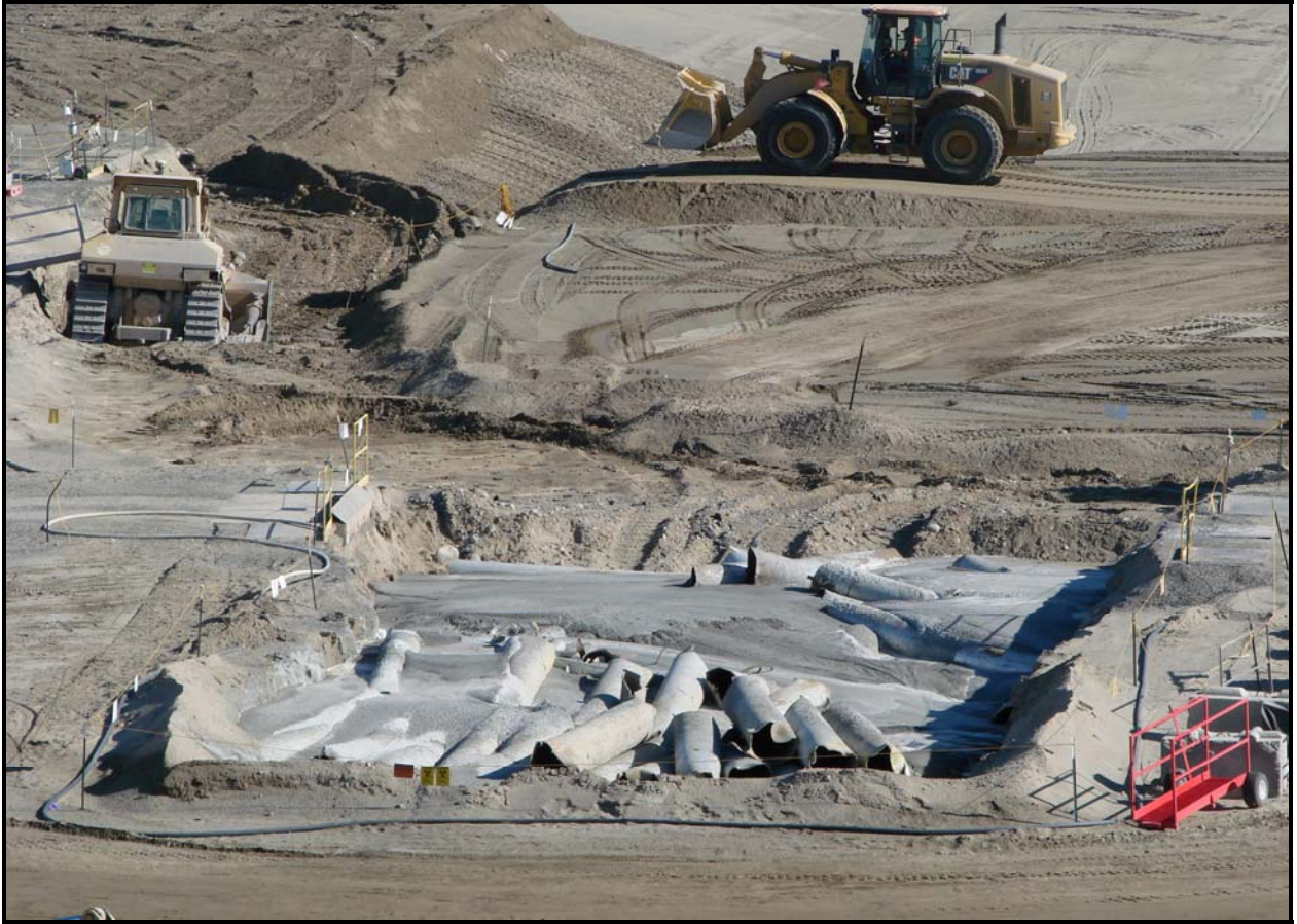
Piping from the water intake structures at K East and K West reactors is disposed in super cell 9 at the Environmental Restoration Disposal Facility. (Photo 2)
