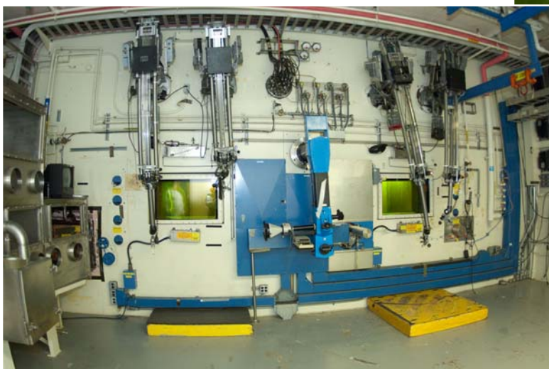
Four massive research labs, or hot cells, have five-foot thick concrete walls with a stainless steel liner. The 324 Building has a Tri-Party Agreement milestone to complete demolition and cleanup in September 2012.
