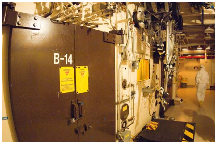
B-cell is the most contaminated of the 3-story hot cell research labs in 324. Experiments included stabilizing high-level radioactive waste into glass.
