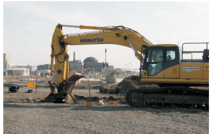
Excavation begins at the first trench in the high-hazard burial ground, 618-1, located at Hanford's 300 Area adjacent to the Columbia River.
