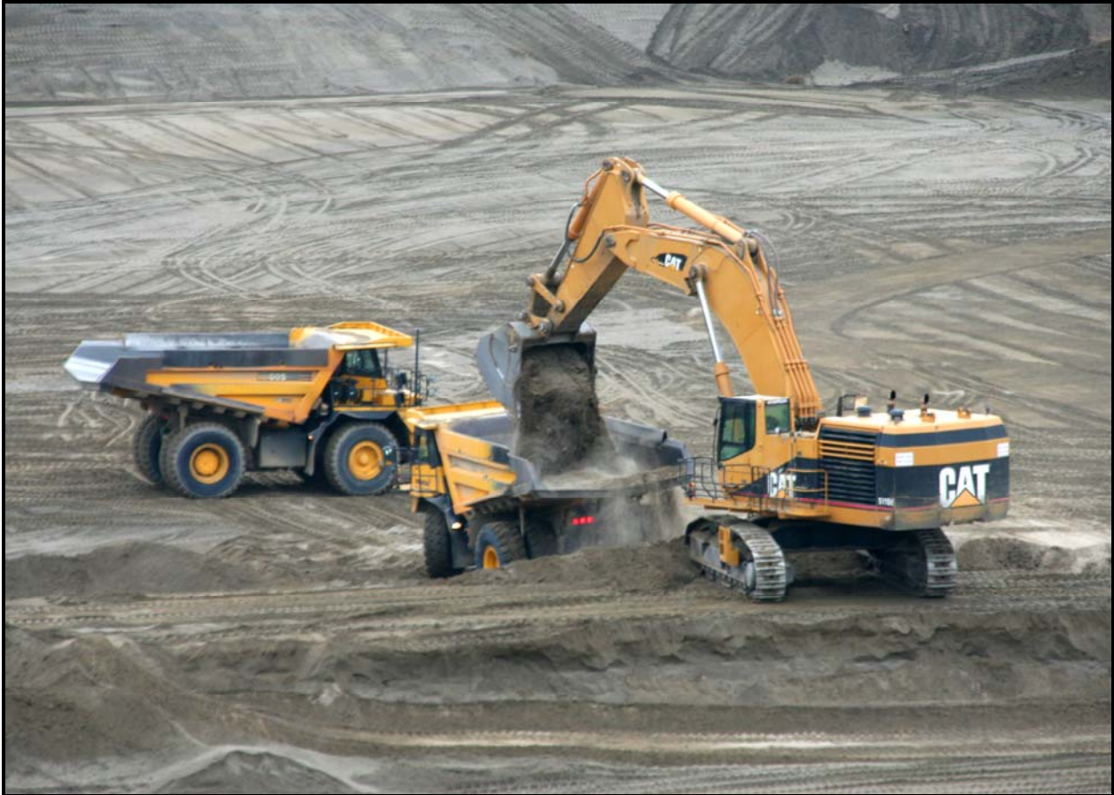
DelHur Industries has reached the specified depth of 70-feet of super cell 9 at the Environmental Restoration Disposal Facility.
