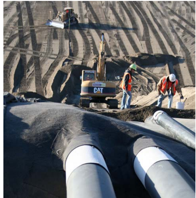
The super cell design features a unique system to collect liquid as it drains through the waste.
