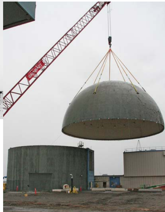
The 67-ton steel dome was removed January 15, 2011. Demolition of the above-grade walls will be completed this winter.
