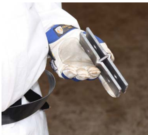
Spacers, called H-clips, were installed after cutting the quarter-inch carbon steel shell off the dome.
