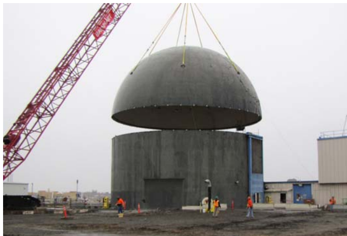
The dome weighs about 67 tons and will be disposed at Hanford's Environmental Restoration Disposal Facility.
