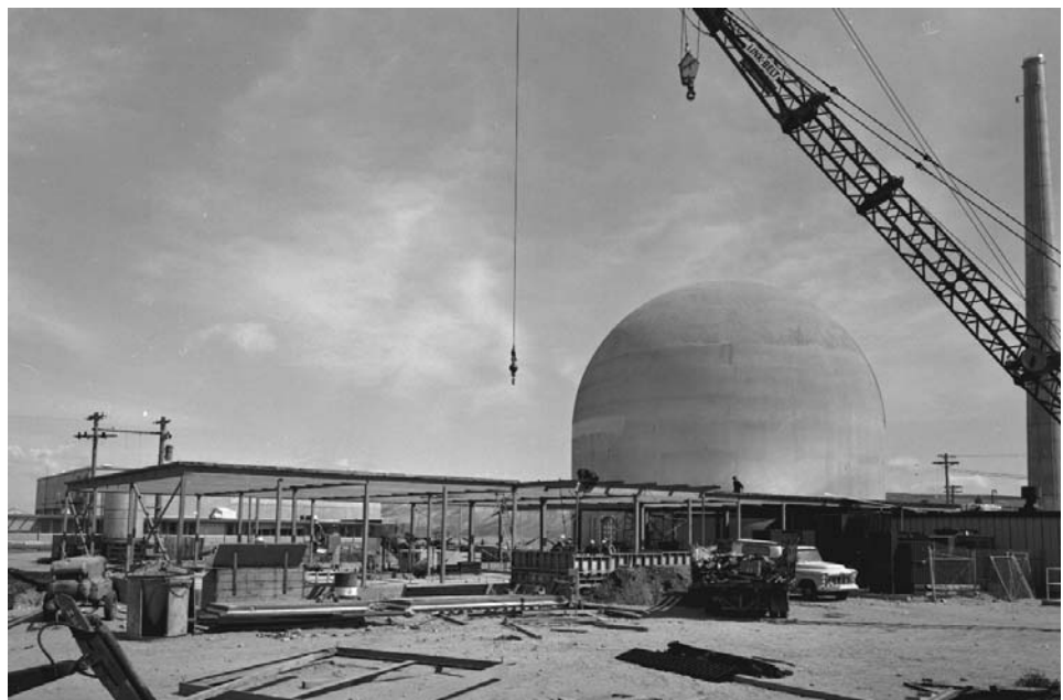
Construction of the Plutonium Recycle Test Reactor was completed in 1960. The reactor operated from 1960-68.
