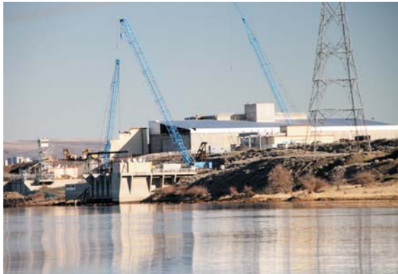
The N Reactor and steam generator buildings are being placed in interim safe storage while workers are cleaning up 119 waste sites at N Area. The work will be completed in September 2012.
