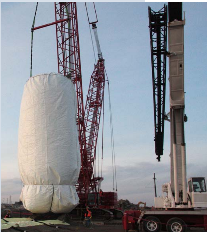
Wrapped in a protective bag that weighs approximately 700 pounds, the CRCTA tank, contaminated with asbestos, was removed from the basement of the 337 Building where mock-up work was conducted for the Fast Flux Test Facility in the 300 Area.
