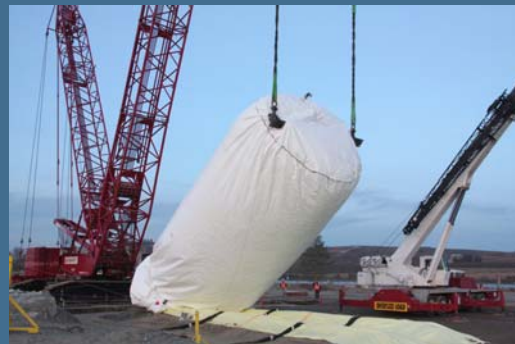
After extensive preparation, the 40-foot long tank is carefully laid on a prepared landing pad.
