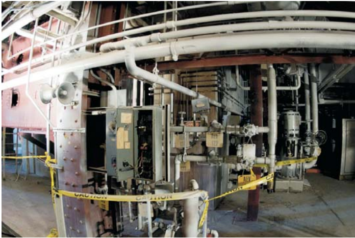
Using explosives on complex and heavy components inside the powerhouse reduces worker risks.
