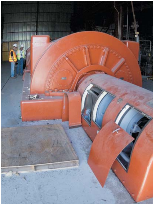
Turbine generator at 184-N
