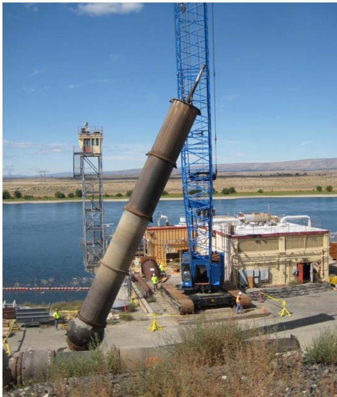
Each river intake structure had four primary electric pumps. Each pump supplied N Reactor with 105,000 gallons of water per minute for cooling water.
