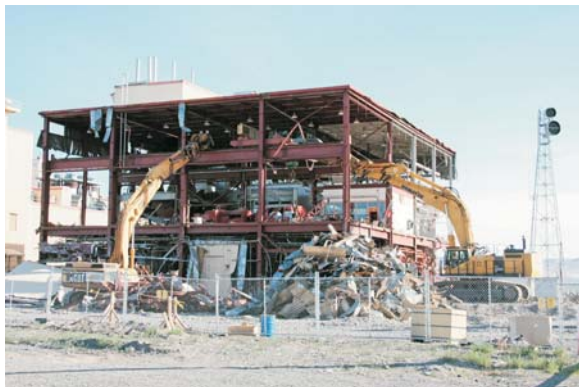
The primary powerhouse facility for the area completed demolition on schedule in September, 2008.
