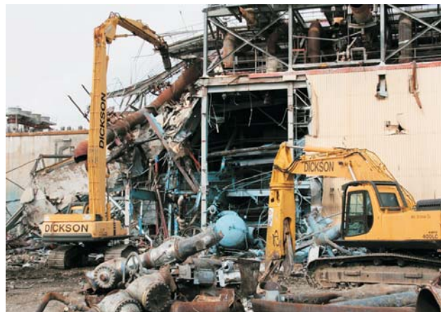
In early April, 2009, the steam generating facility demolition nears completion up to the four-foot-thick shielding walls surrounding N Reactor's core.
