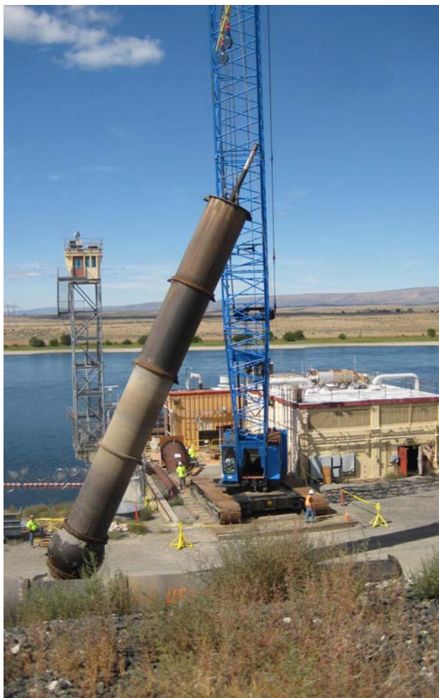
The water intake pump is 60 feet long and provided 105,000 gallons of water per minute to the reactor.
