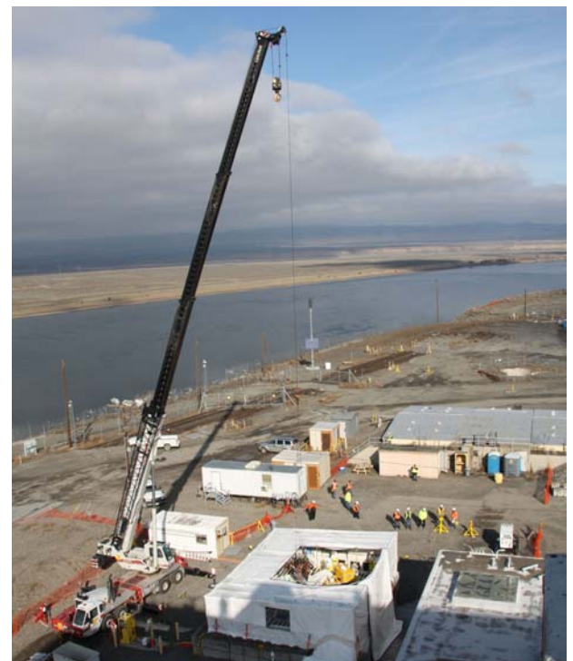
A fission product trap cyclone separator is removed for packaging and disposal, February 2010.
