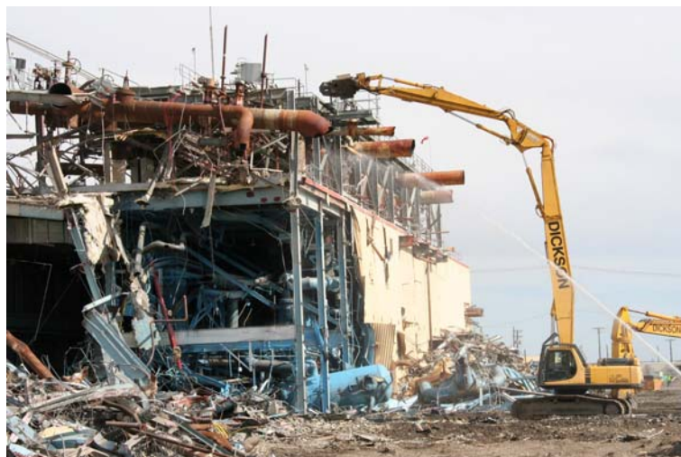
Demolition of the Heat Exchanger Building, 2009. N Reactor was the only facility in the U.S. to produce plutonium and steam for electricity.
