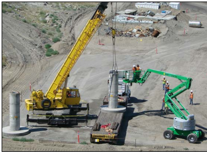
Disposing of Interim Storage Vessels
