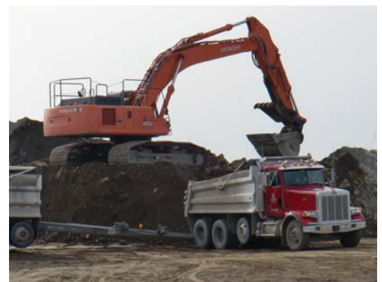
Phoenix Enterprises NW uses its own truck and pup outfit to load out material at the IU 2 & 6 project.
