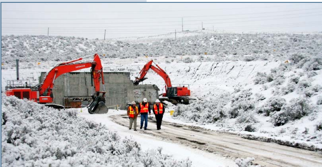
Field Remediation workers just completed excavation of the old plutonium vaults on Gable Mountain. The vaults were built into the hillside and were used to store plutonium before it was shipped offsite. Later, it was used to store explosives. A culturally sensitive area, the site will be restored to its original state, including removal of the access road. Pictured are George Dvorak, FE&C, and Ernie Biebrich and Robert Gray, WCH.
