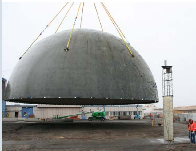
After size-reducing, the dome’s new home will be Hanford’s Environmental Restoration Disposal Facility.
