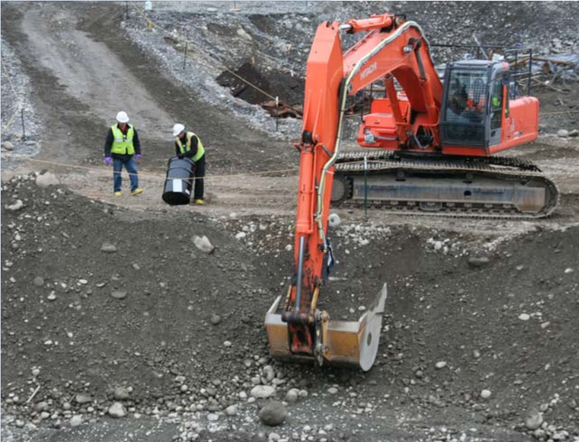
Cleanup of the 118-K-1 Burial Ground resumed in January 2010. Workers expect to remove an estimated 370,000 tons of contaminated material before the project is completed in December 2012.
