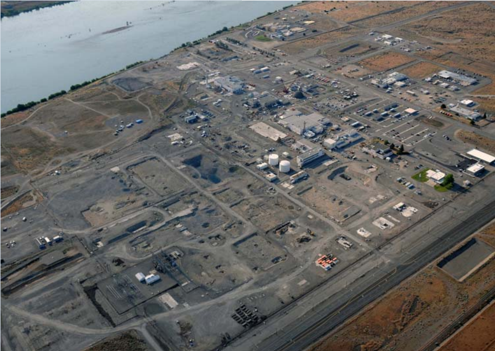
A closure team is finalizing plans and initiating the challenging final cleanup activities in the 300 Area by the end of the river corridor closure contract. This June photo shows tremendous change at Hanford's 300 Area along the river corridor.
