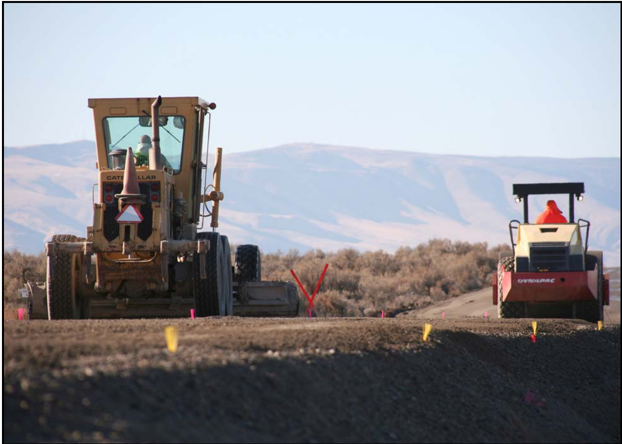
Richland subcontractor George A. Grant continues work in preparation of paving the back road to the Environmental Restoration Disposal Facility.
