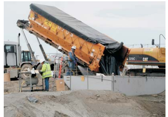
Scott Sutton and Gunnar Leidel, with Stoller, dump lead-contaminated soil into a mix box. The lead-contaminated soil is mixed with cement as part of a treatment process and must be removed before it hardens. The crew will treat about 28,000 tons of lead-contaminated soil from the 618-7 Burial Ground over the next two months.
