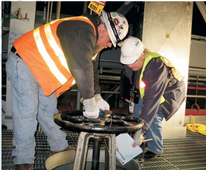
Charles Reed, left, a laborer with the Wm. Dickson Co., removes one of six seals from steam valves in the 109-N Building. Nancy Maguire-Moffitt of PNNL, will give the seals to members of a Russian delegation who monitor compliance with the Plutonium Production Reactor Agreement.
