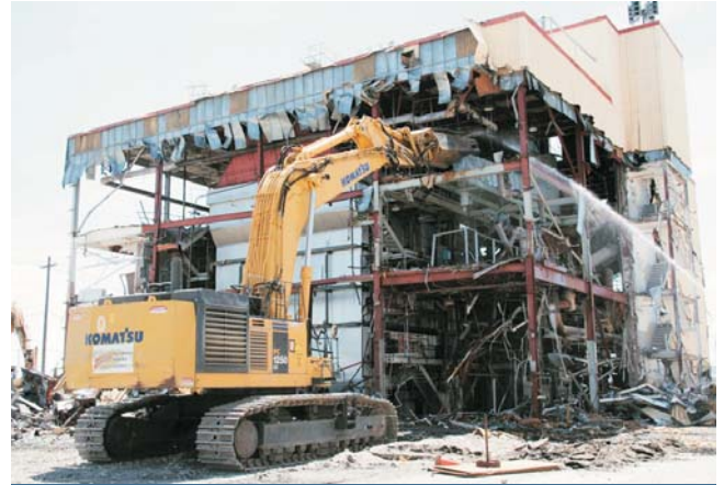
D4 crews dismantle piping and equipment in the 184-N Powerhouse in the 100 Area. The work was completed on time and met a September TPA milestone.
