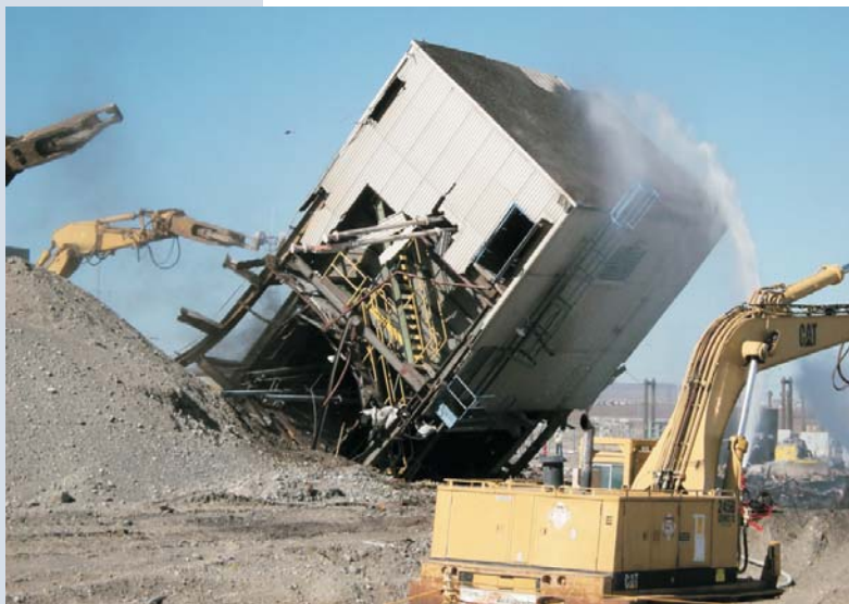
The successful demolition of the 384 high bay in the 300 Area overcame numerous challenges in 2008.
