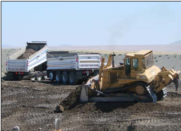
Disposing Soil from 100-D in Cell 6 70-ft Level Using Truck and Pup Operations
