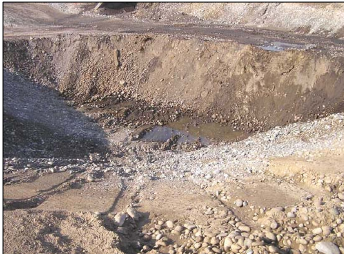
Groundwater Found in Bottom of Excavation at 128-H-1 Burn Pit
