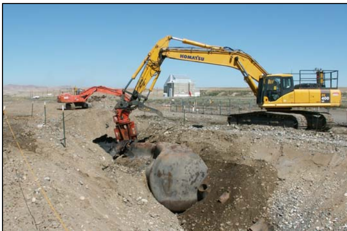
Shearing Open Railcar at 118-F-2
