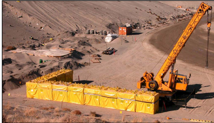
Eleven K-Basin Ion Exchange Modules Staged on the 35-Foot Level of ERDF Cell
