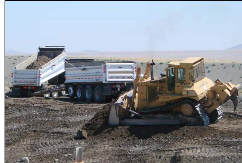
Disposing Soil from 100-D in Cell 6 70-ft Level Using Truck and Pup Operations
