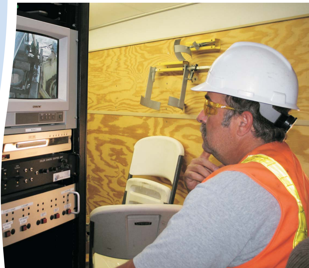
Keith Tarr of subcontractor Federal Engineers and Constructors operates the remote saw from the surveillance trailer before workers drain unidentified materials from the tubes excavated from the site.
