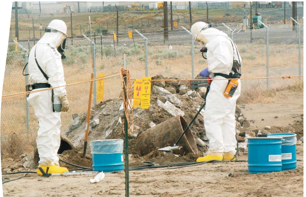
Envirocon employees' effort to clean up the 618-2 Burial Ground is just one example of work subcontractors are performing in the 300 Area.
