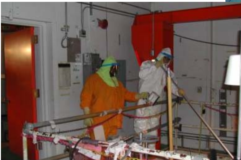
Workers apply a fixative to a nuclear fuel storage basin inside 327. Fixatives were utilized extensively throughout the entire building to control the spread of hazardous PCBs, asbestos, beryllium and high levels of radiological contamination.
