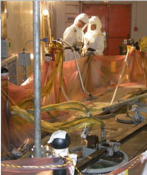
Workers use diamond wire saws to cut hot cells free from the cement floor.
