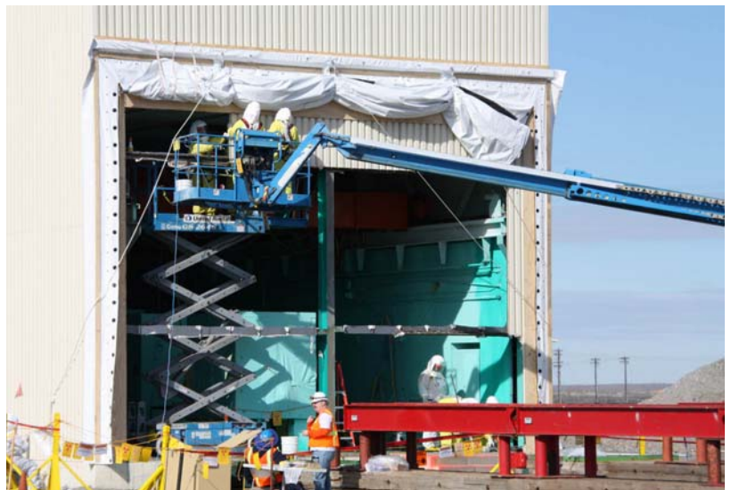
Workers prepare an opening in the exterior wall where the hot cells were rolled out with a gantry system.
