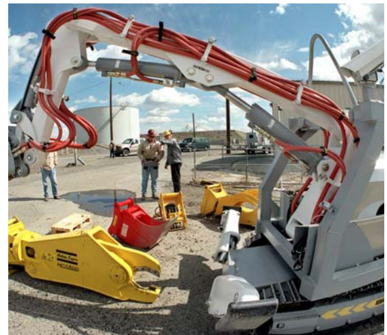
The Brokk was used to remotely cut loose contaminated pipes and equipment so the 10 hot cells had clearance for removal from the building.
