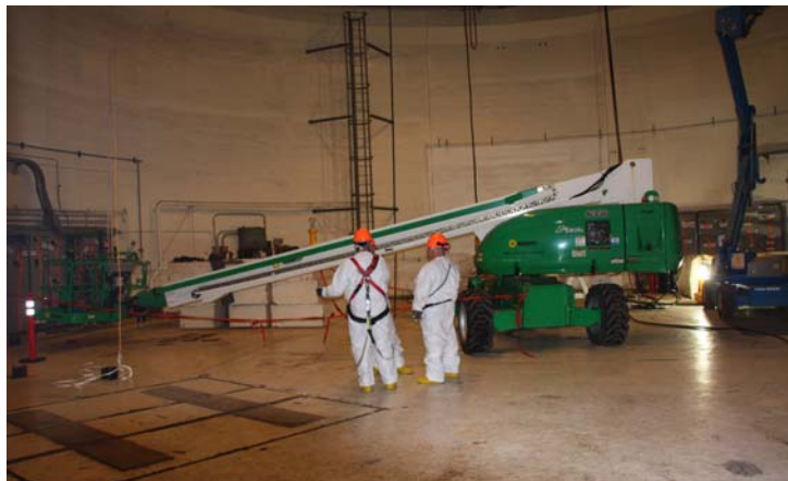
Inside the 309 Building, months of preparation were required to remove hazardous materials and to stabilize the dome before demolition.
