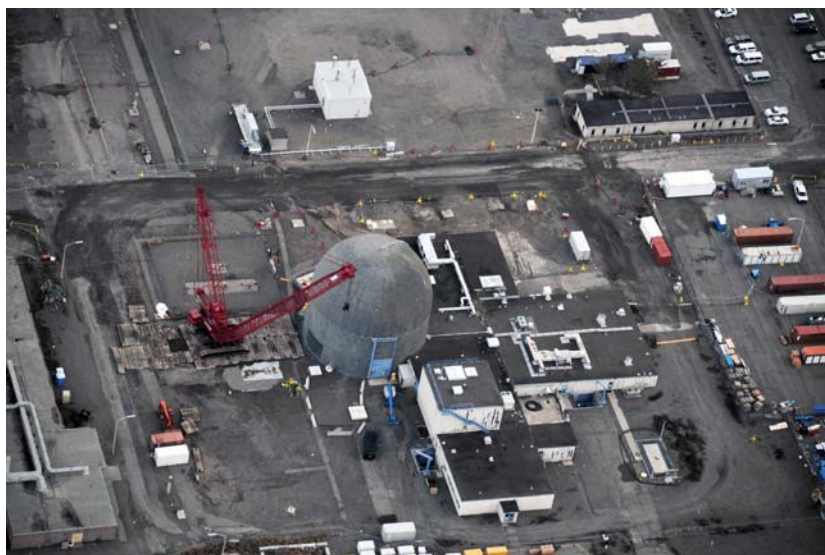
The crane used to remove the 80-foot-tall dome has a 200-foot boom and weighs 500 tons.
